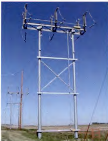
Steel H-frame structure with airbreak similar to the proposed
